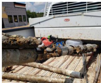
10 clamps from previous repairs
